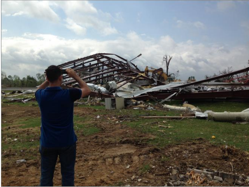
Figure 5.15 A ground photo for a metal building severely destroyed and rated as EF4 at location (R2L3), Taken by UA team.
