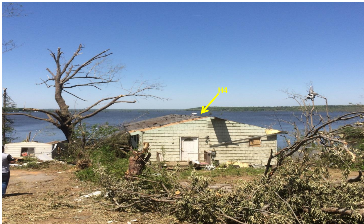
Figure 4.23 Minor roof damage (EF1) for the house (H4) on the leeward side (low elevation 83.8 m (275 ft)). (UA team photo).
