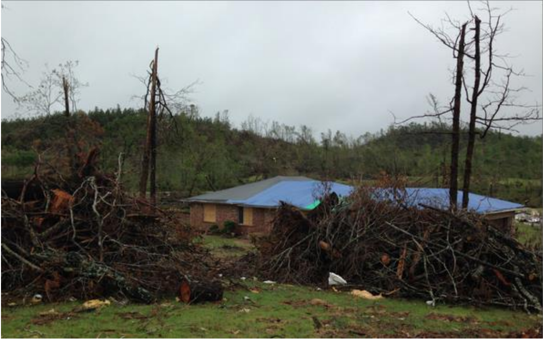
Figure 5.7 A house in location (R1L2) with a little damage to the roof rated as EF1, taken by UA team.
