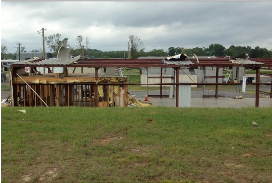
Figure 5.16 A metal at location (R2L3) harshly damaged, almost all the sheets are detached and many columns and beams are bent, Taken by UA team.
